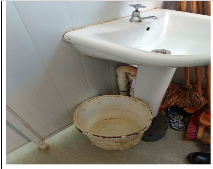
Figure 12: Bucket used to flush grade 1 toilets due to low pressure (Researcher, 2024)
