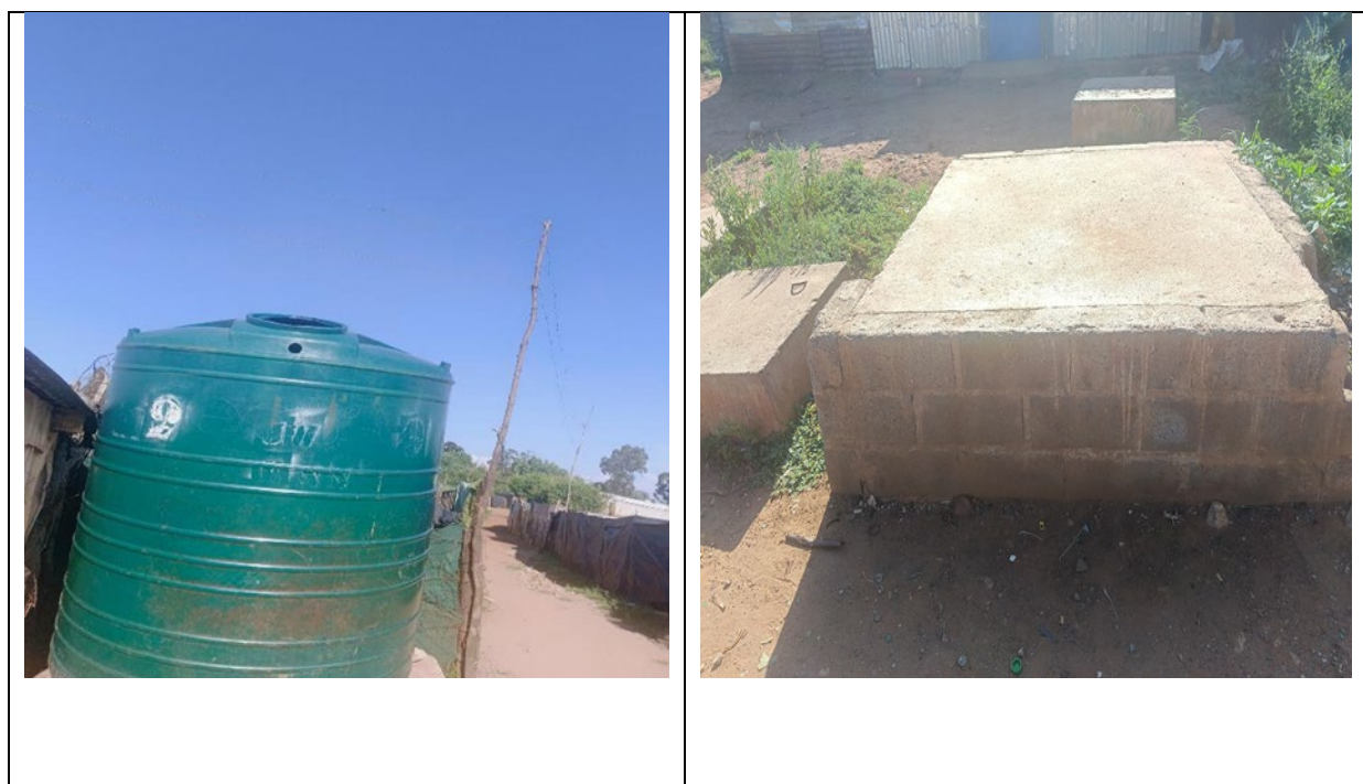
Figure 17a and 17b: Tank 7 with no top lid. Source: Researcher (2024) and Tank 3 (Stolen tank). Source: Researcher (2024)
