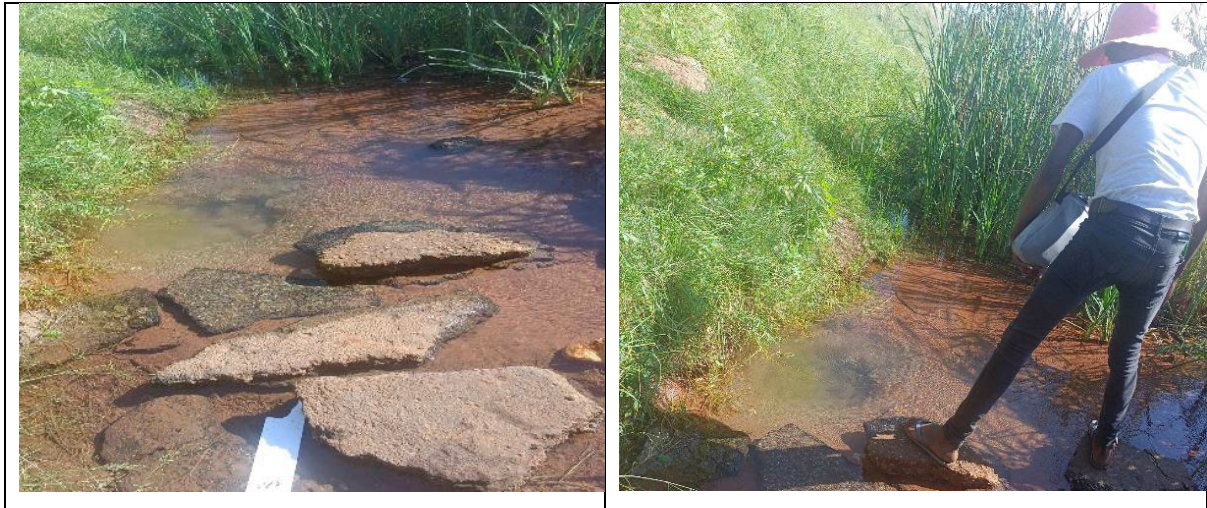
Figure 19a and 19b: Underground leaking pipeline Source: Researcher (2024)
