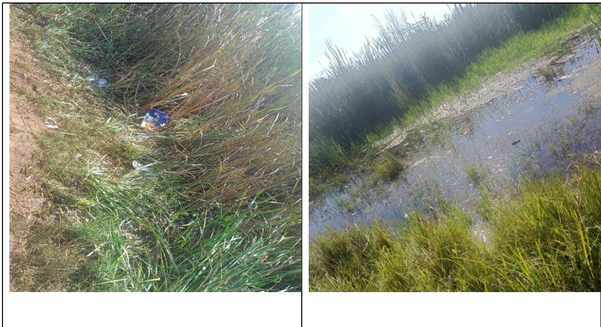
Figure 20a and 20b: Evidence that people do their laundry at the leaking pipeline. Source: Researcher (2024) and Pond with polluted water. Source. Researcher (2024).
