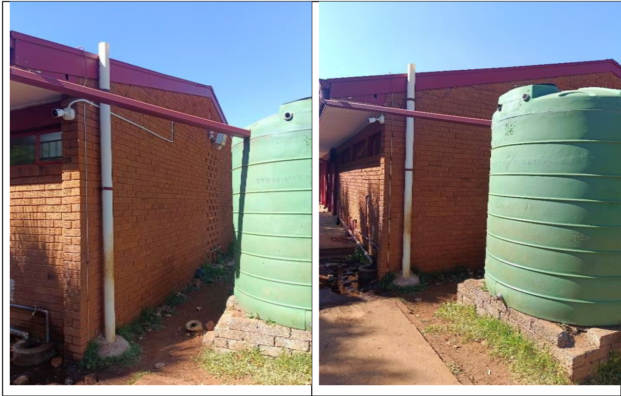
Figure 10a and 10b: Water tanks used for rain water harvesting (Researcher, 2024)
