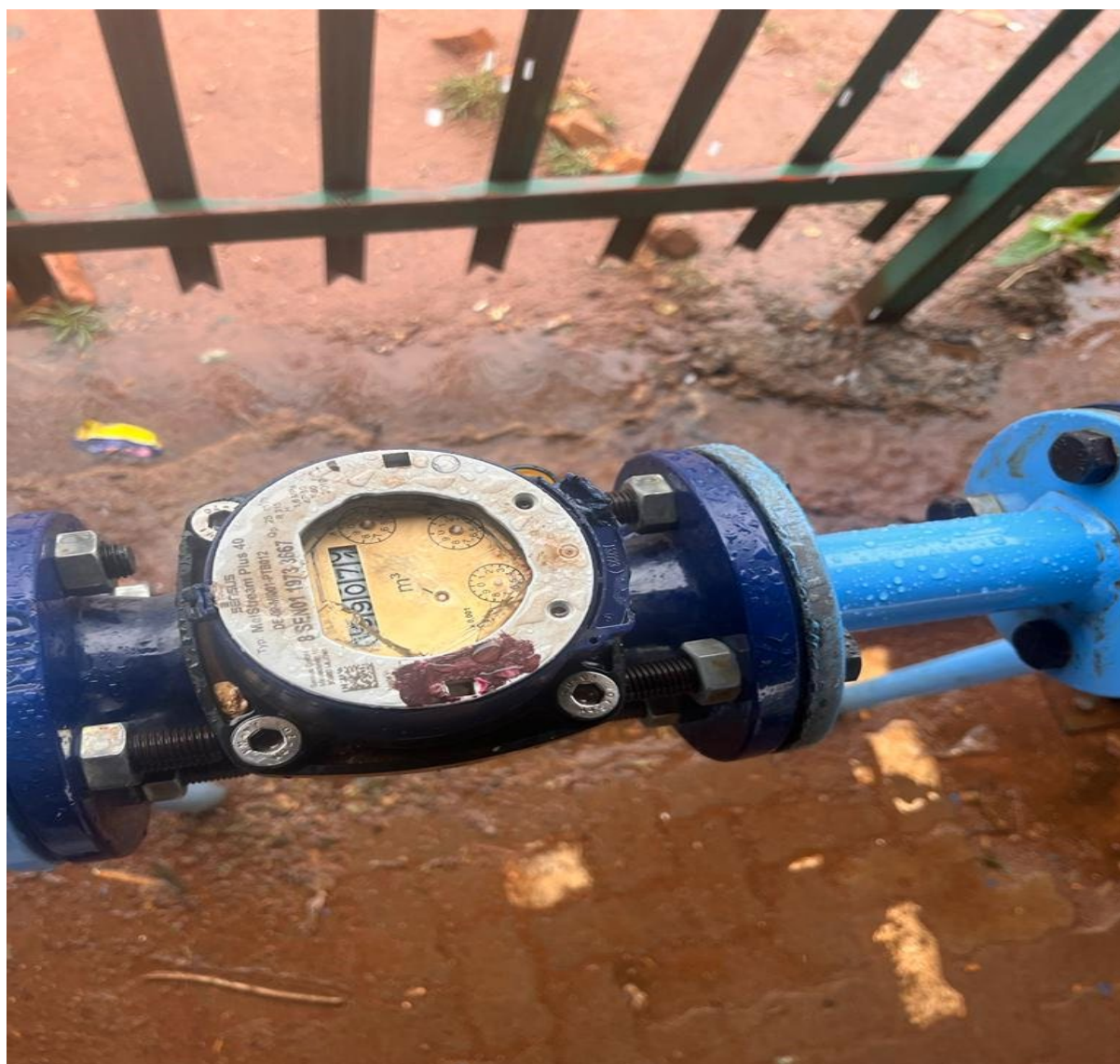
Figure 4.4: Broken water meter at school A. (Photo: Mndawe. S, 26 October 2023).
