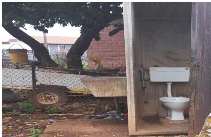
Figure 15: A picture showing a malfunctioned toilet in the Shawela informal settlement (picture by researcher)
