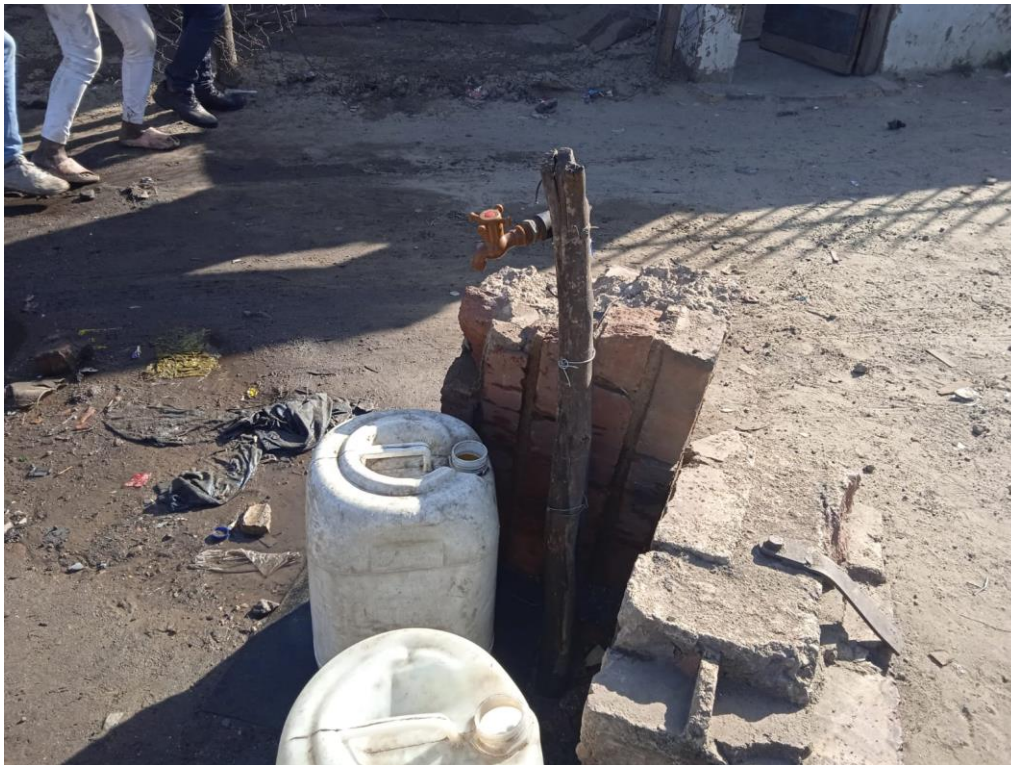
Figure 7: Broken and leaking taps, Nkuna, 2023.
